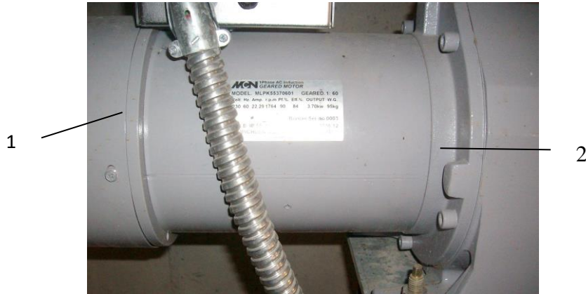
Fig. 2. The conveyor’s motor. 1 – motor; 2 – flange
